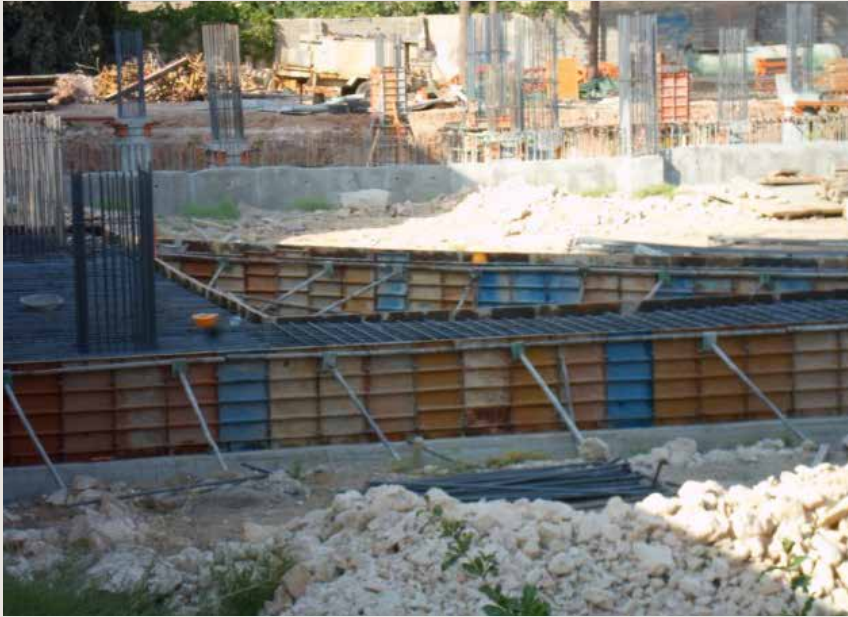
A photo of ongoing construction work at the Bahá'í cemetery in Shiraz, where the Revolutionary Guard has been building a "sports and recreation" complex since April 2014.
